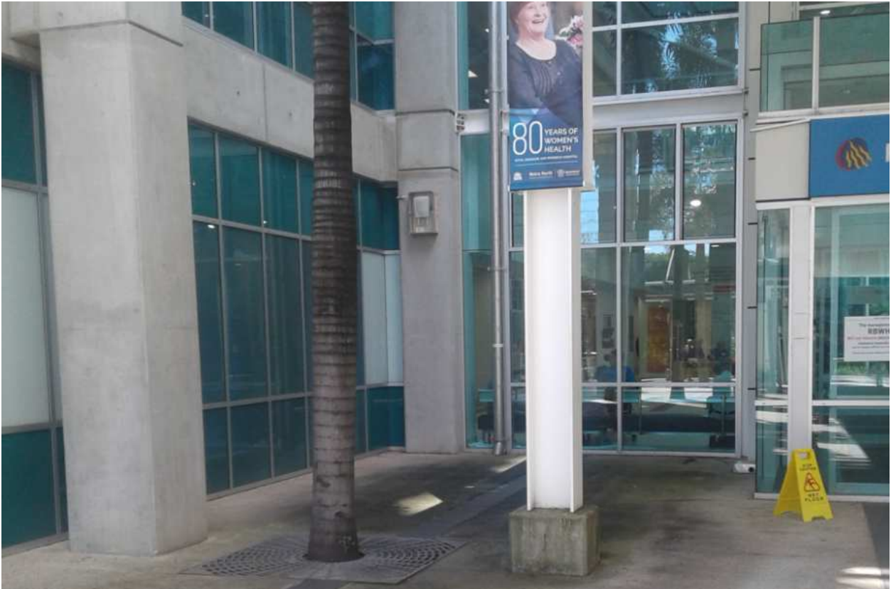
Figure 3 - Dead space beside main entrance doors. Space does not appear to impede fire egress under NCC
